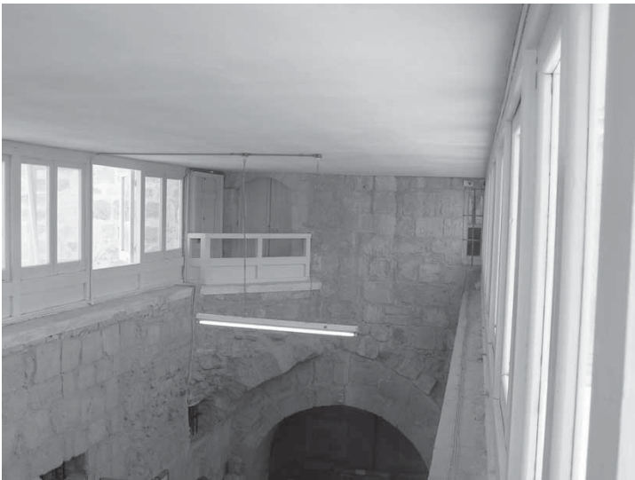
Fig. 40: Limassol Castle, roof level, eastern roof chamber doorway above remains of barrel vault [M. Olympios].
